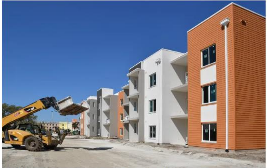
The Sarasota Housing Authority is nearing completion on Cypress Square, a three-building, an affordable housing project consisting of 84 units and a clubhouse in the 1800 block of 21st in Sarasota. Mike Lang
